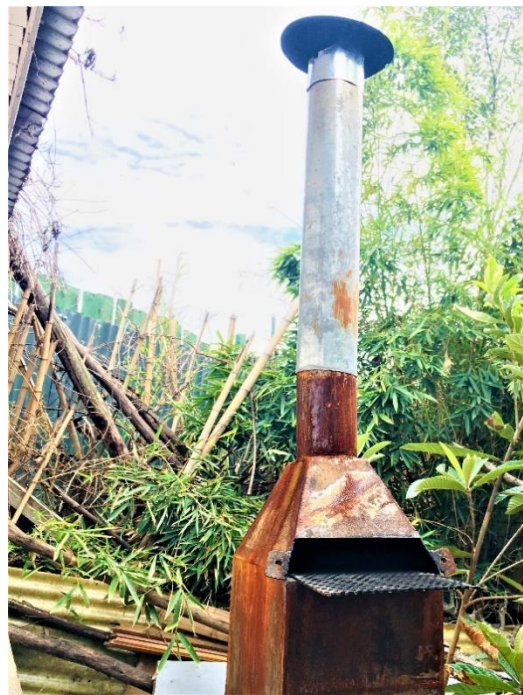
Figure 21: Chimney and smoke treatment chamber assembly
